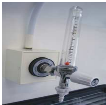
Figure 7.5: Example of Oxygen Panel
